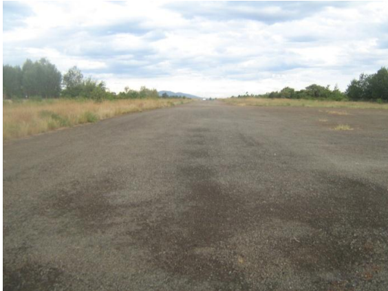
A view of Embu Airstrip located (332104E;993739N) East of proposed Embu substation
