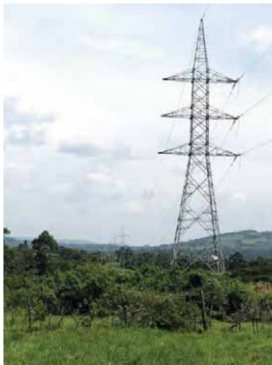
Plate 1: Typical design of a steel lattice type transmission tower
