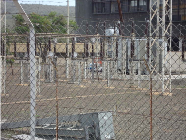
Fig.3.3: Geo-thermal Power Station's switchyard where the proposed line will originate
