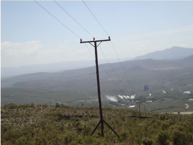
Fig.3.4: Existing 33kV Line at Hell's Gate National Park The line passes through the following areas;
