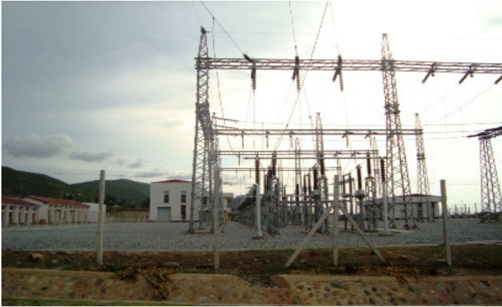
Fig. 3.13: Sondu Miriu Power Station
